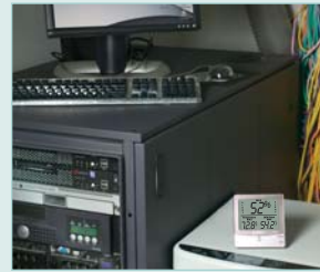
Alerts low Humidity levels in Computer rooms to help prevent electrostatic conditions.
