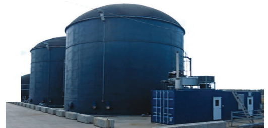
Figure 22.6 Sludge digestion tanks.
