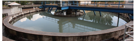
Figure 22.5 Secondary sedimentation tank.
