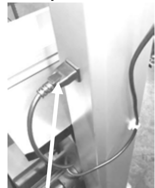
Light plugged into 110v socket
