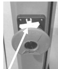
Start/stop with safety removed
